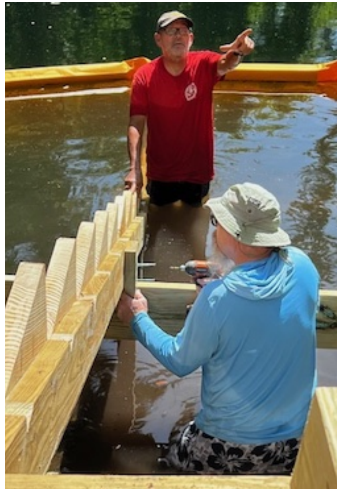
RB Havens and Tom Johnson install stringers during the May 2025 project to replace the lower set of stairs at Orange Grove. Photo by Fred Stratton.
